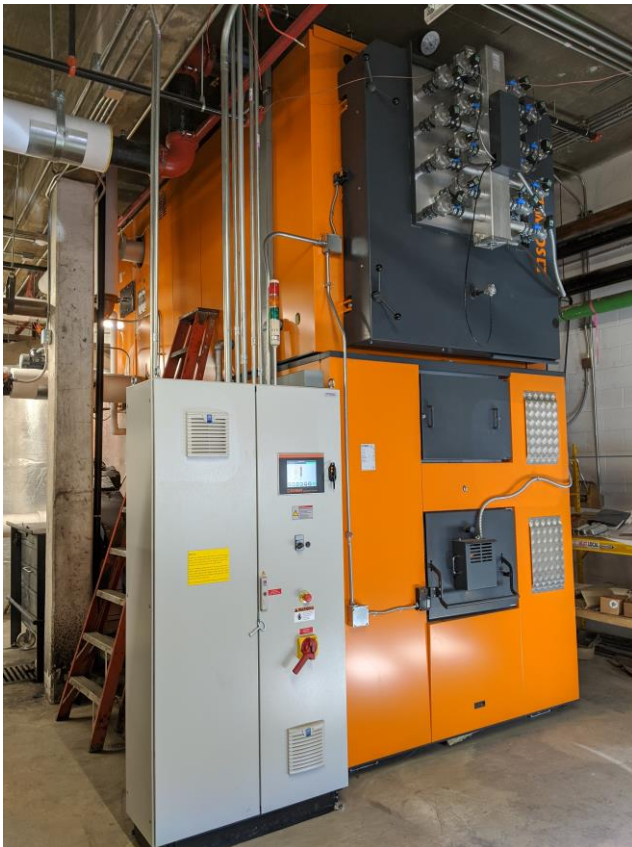
Maplewood Nursing Home Wood Chip Boiler
