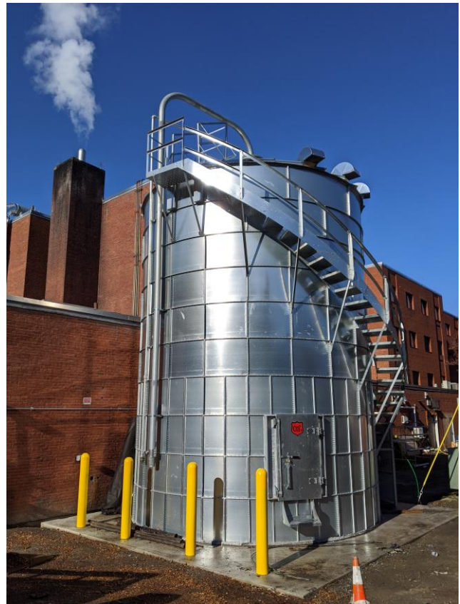
Wood Chip Storage Silo
